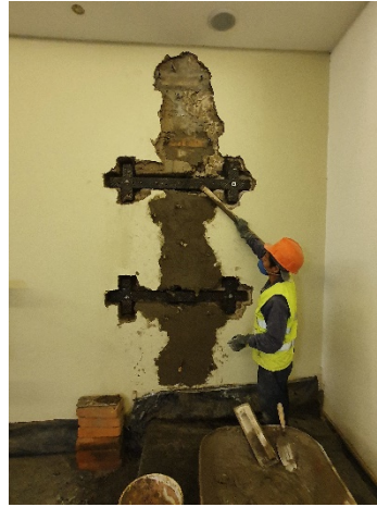
Figure 17 Wooden key image protected with asphalt paint and wrapped with mesh. Anchoring with steel rod
