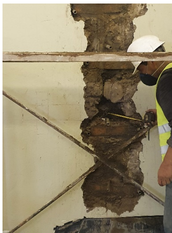
Image of the process of unpicking and stitching of the affected masonry
