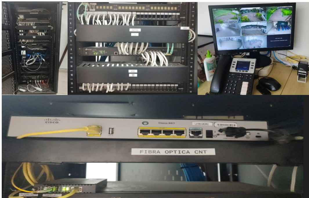
Figure 3 Telecommunications Technology Equipment
